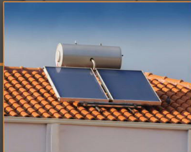
Solar Water Heating
